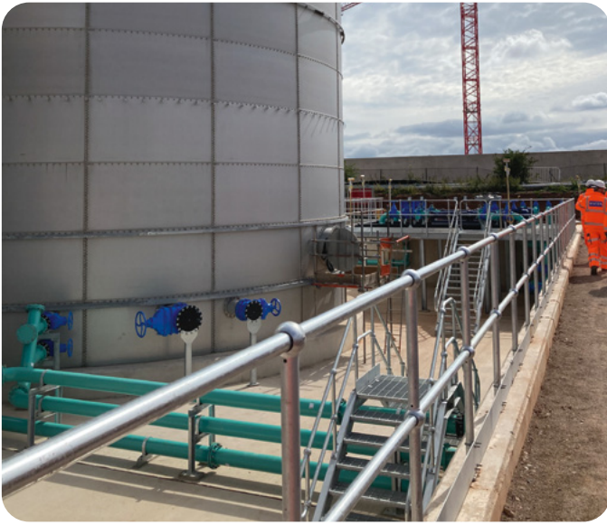
Wanlip Sewage Treatment Works, Leicestershire
