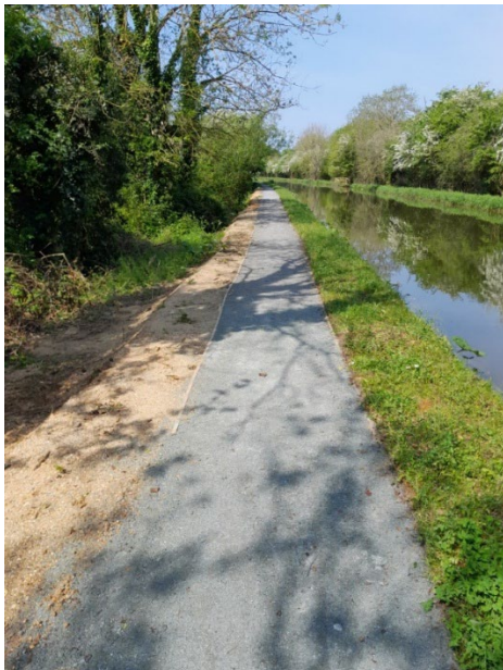
Figure 2.4. Example of completed bank raising work recently carried out by the Trust
