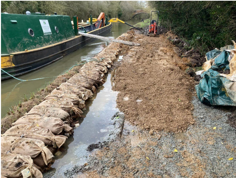
Figure 6-5 Photograph of an Example of Raising Works Showing Access (Reproduced with kind permission of the Canal & River Trust)
