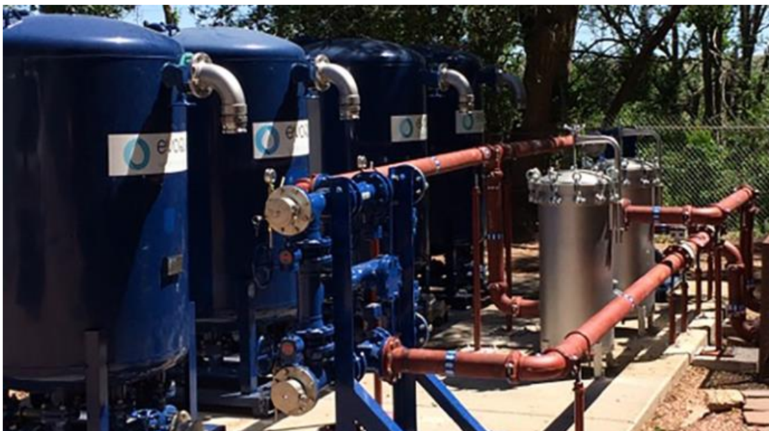
Figure 6-1 - Ion Exchange Vessels (Evoqua)
