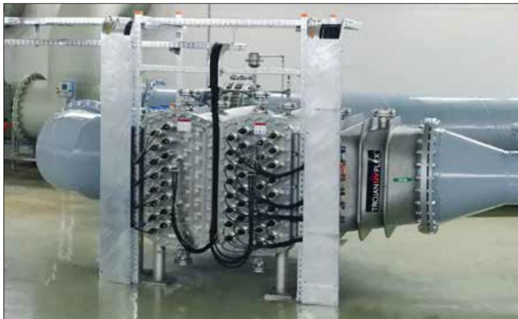
Figure 7-1 - Modular UV Chamber (Trojan)
