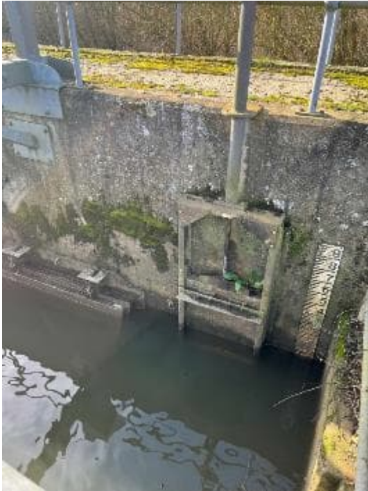
Plate 63 Sluice gate controlling outflow of Hemington Brook to the River Soar
