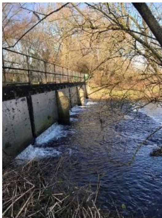
Plate 23 Sluice gates controlling outflow of Main Pond to the River Trent
