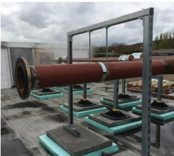
Figure 6-6: Example of a type of pipe clamp arrangement
